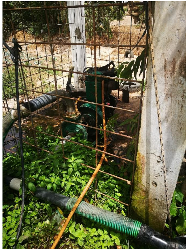
Borehole (with electric pump)
